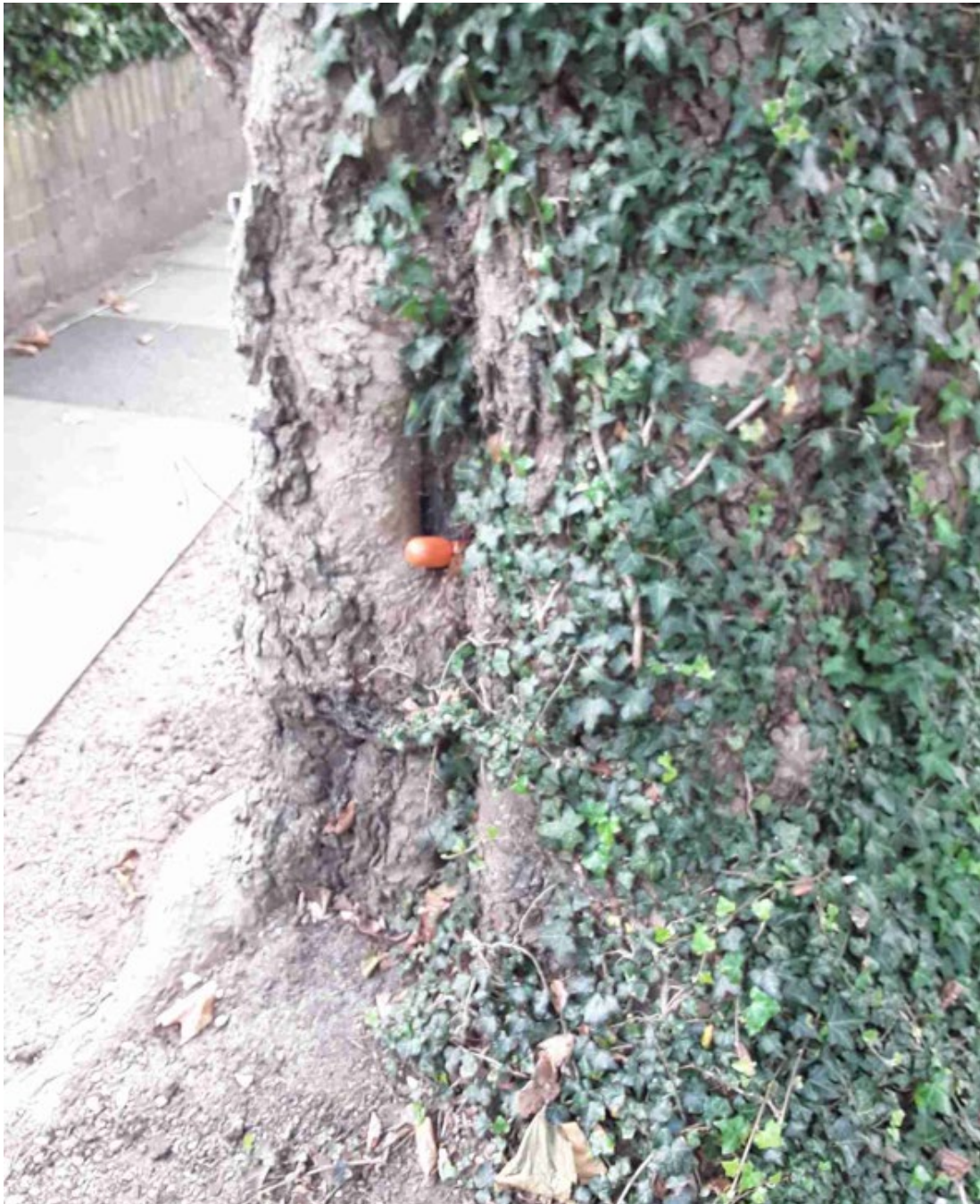
Image shows decayed area of the stem of the tree (end of orange probe visible in photo)
