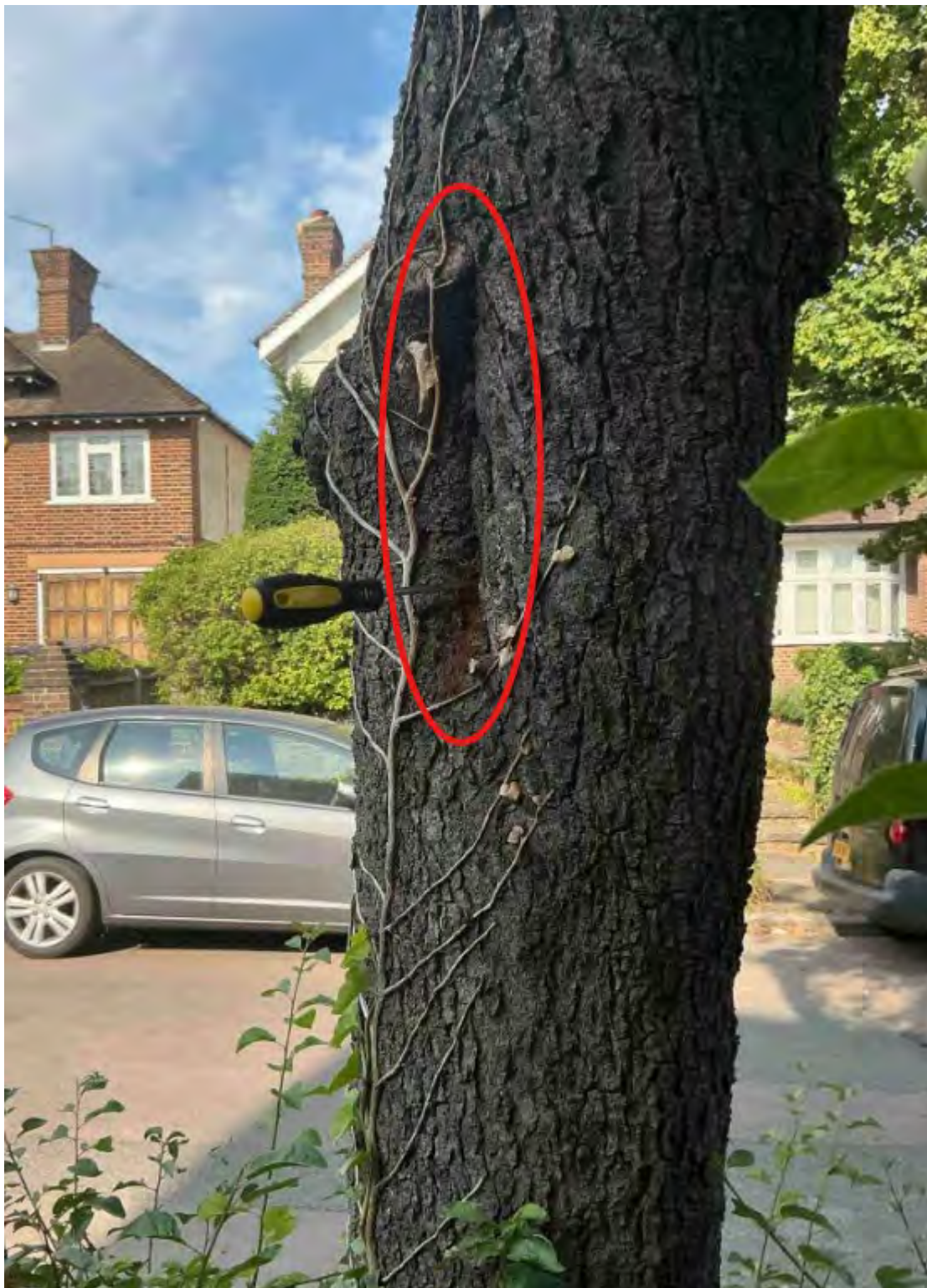
Image shows cavity on trunk circled.
