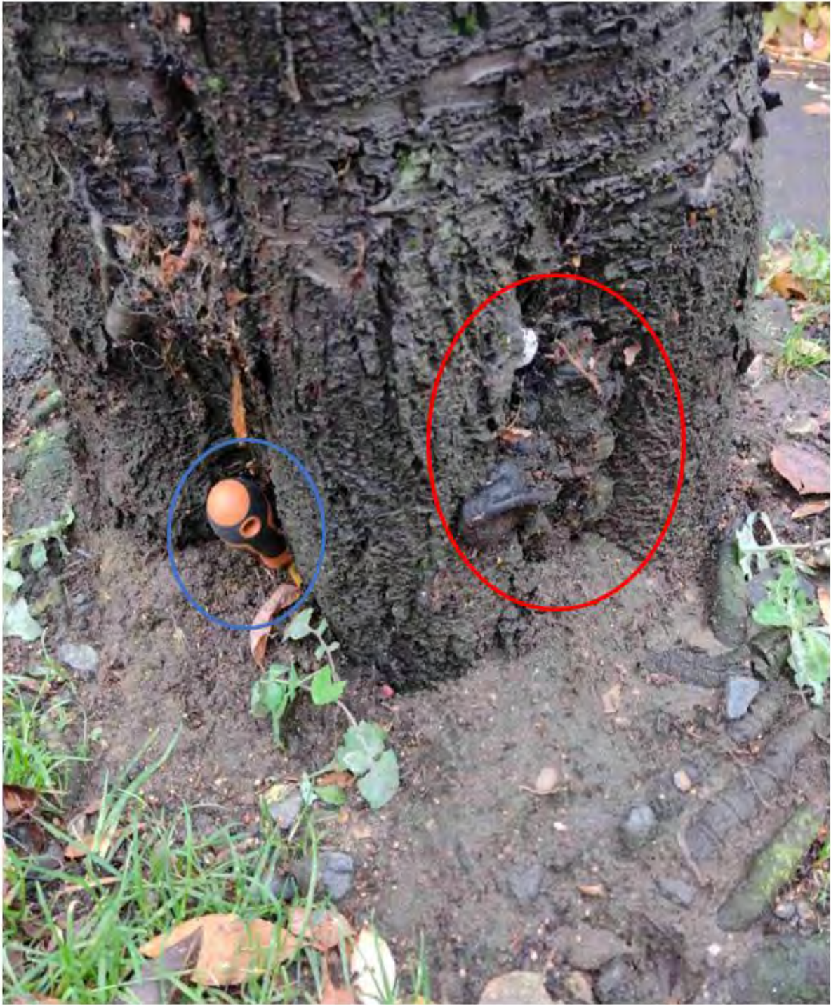
Image shows Ganoderma circle in red and probe circled in blue highlighting decay in stem.
