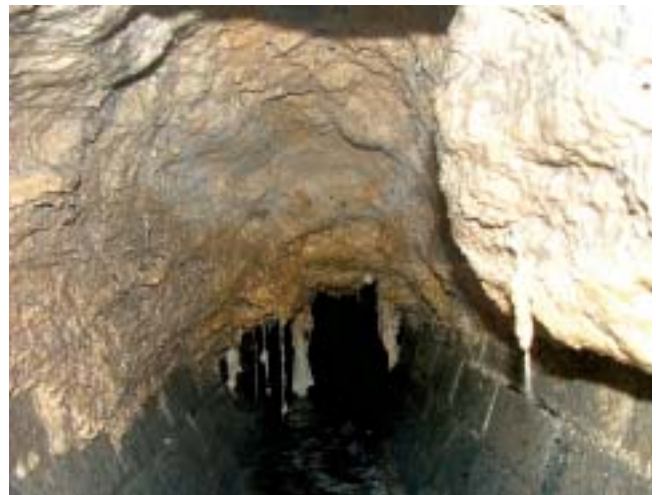
Fat beginning to block a sewer
