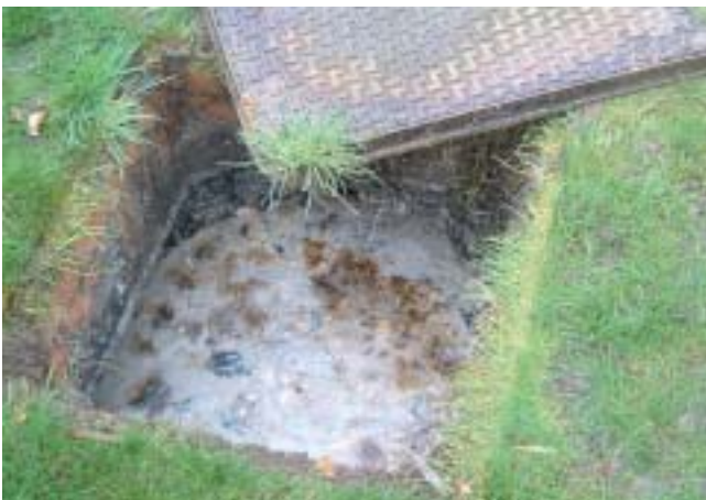
Fat building up in a manhole
