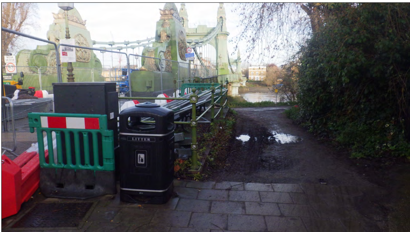
Plate 3: View of position of the southern abutment to temporary bridge (looking north) with Hammersmith Bridge in the background
